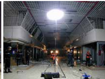
Securing a shopping mall after an explosion
